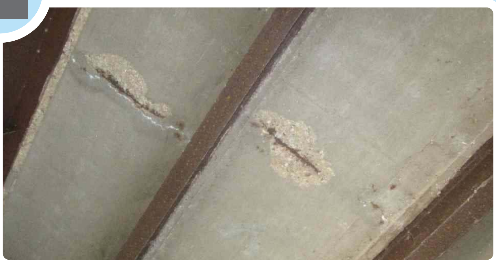
Concrete on the bottom of the bridge deck is cracking and chipping off, exposing the reinforcing steel.
