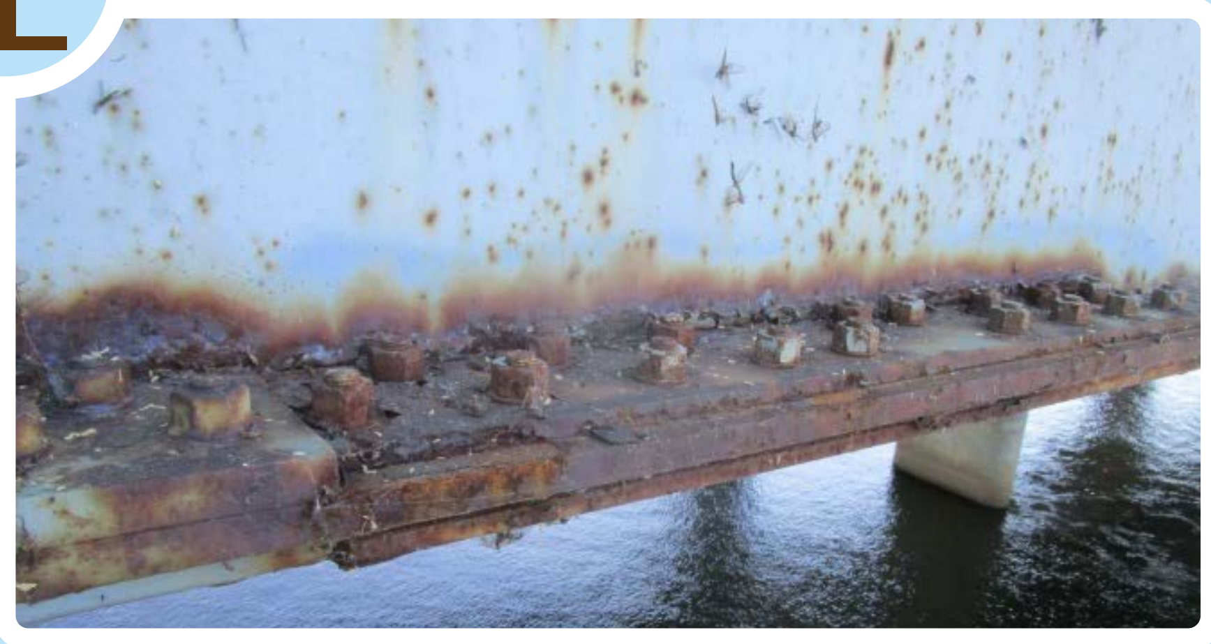
Loss of protective coating over steel elements and connections.
