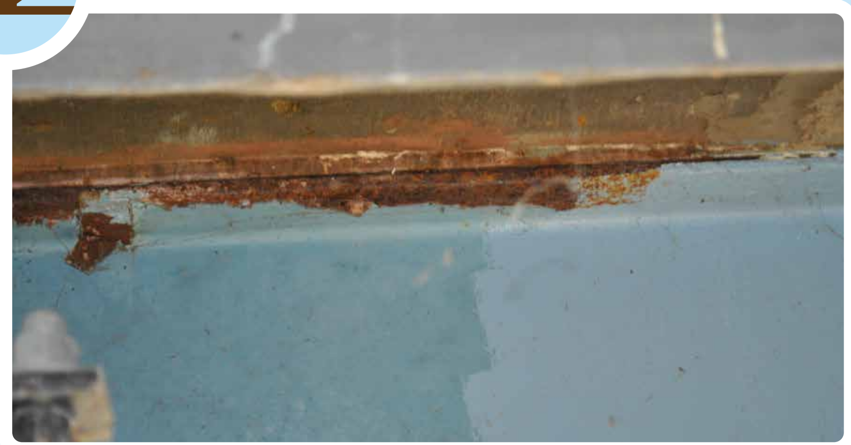
Pack rust has formed between steel elements causing bulging and distortion, leading to added stress and cracking in the concrete deck.
